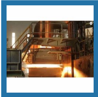
Ladle Refining Furnaces
